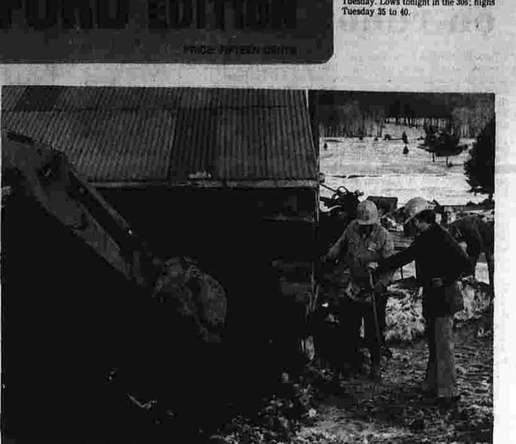
Charles Sheehan, right, talks with construction supervisor Ted Cowing of R.J. Alexander Inc. of East Hartford on the site of the new East Hartford Golf Course garage off Long Hill Street. The sun was sinking Friday as the firm's equipment sunk into the ground to meet a federal funding deadline. (Herald photo by Barlow)
